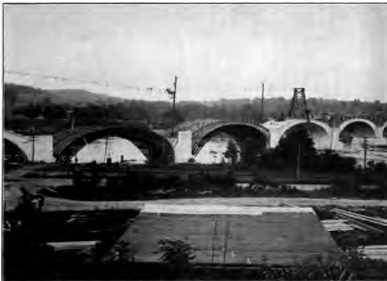
THE LACKAWANNA IS BUILDING THE LARGEST CONCRETE BRIDGE IN THE WORLD ACROSS THE DELAWARE RIVER AT SLATEFORD, PA.
